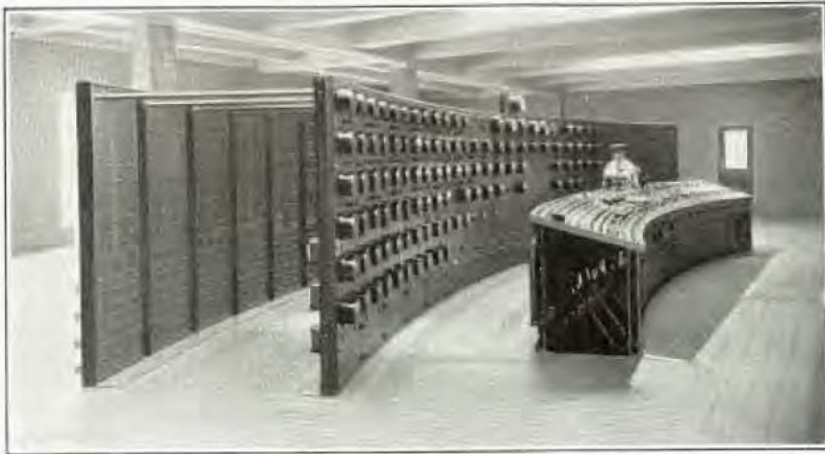
The Switch-board in the Power Plant at River Rouge
