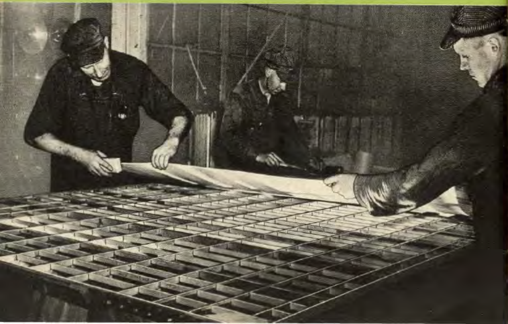
These men formerly built station wagon bodies at Iron Mountain. Here they have the task of building the glider's floor structure. Honeycomb design adds greater strength with less weight.
