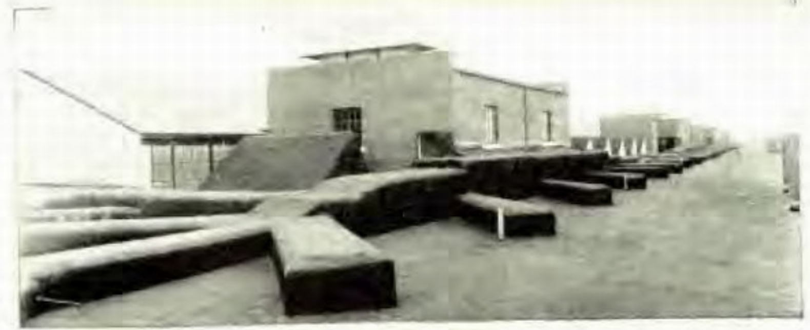
Roof Heating System
