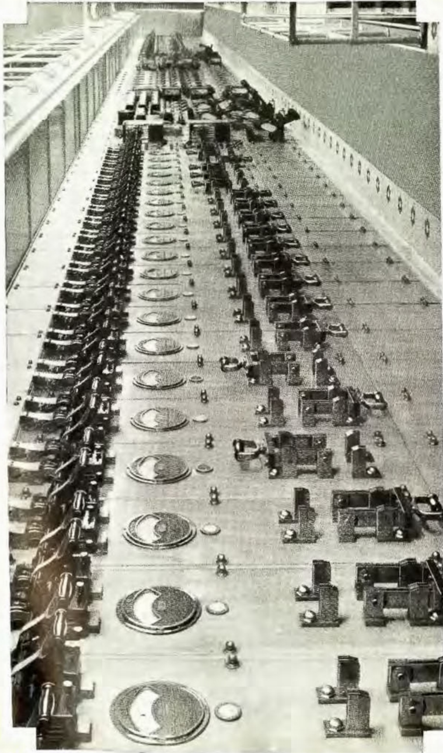
The Power House Equipment Includes the Largest Direct Current Control Board in the World
