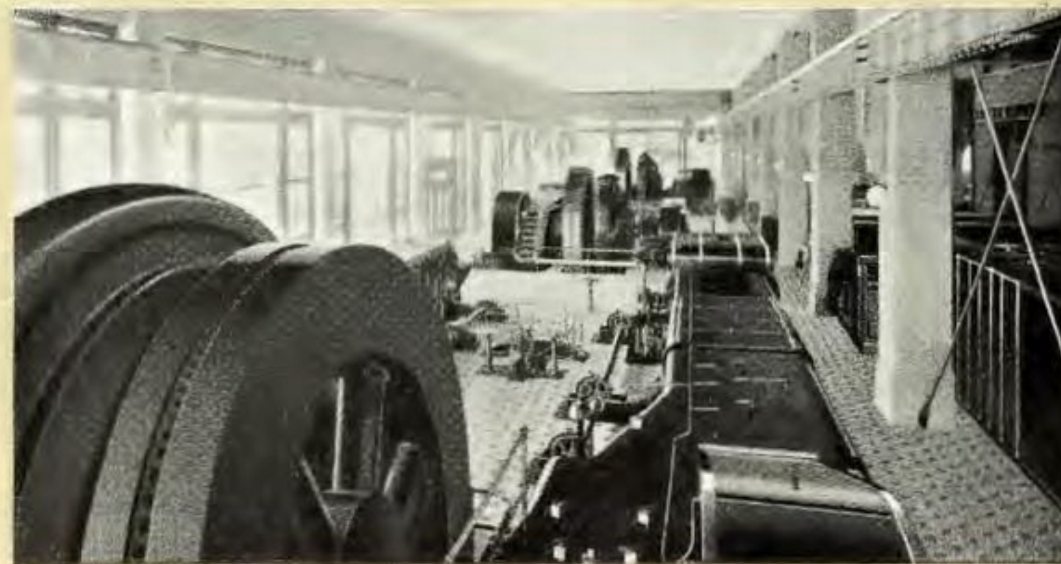
6,000 h. p. Gas-Steam Engine—Showing Flywheel and Electric Generator
